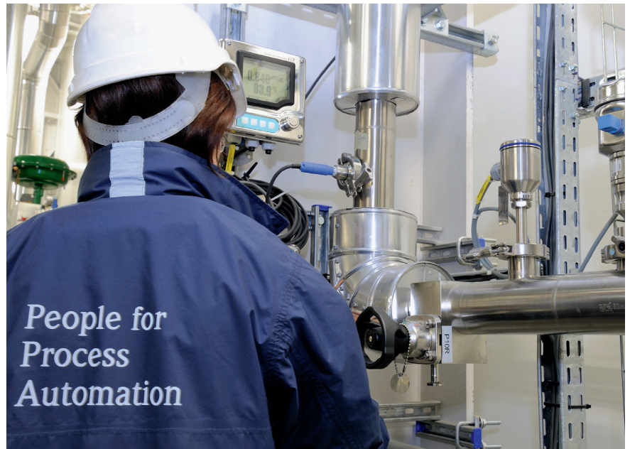
Endress+Hauser GMP trained technician during an inspection of a WFI loop.
